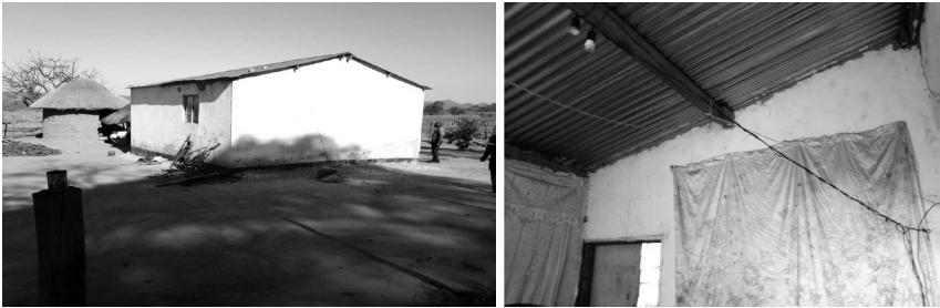
Illustration 2: Houses constructed for community in Zvishavane (crack on top of the wall on the right side)
